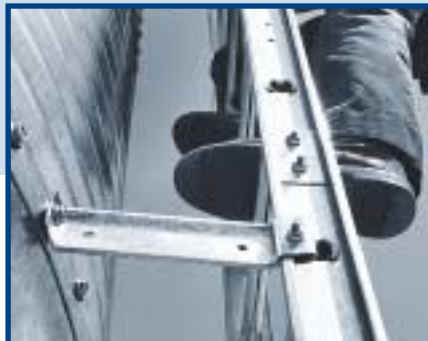
Side ladders allow plenty of space between rungs and bin wall for a secure footing.
